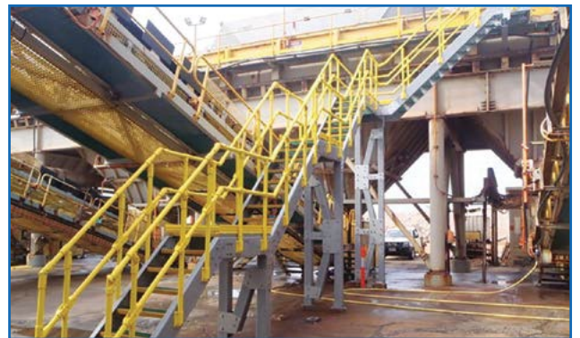
FRP Handrail and walkway
