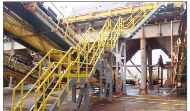
FRP Handrail and walkway
